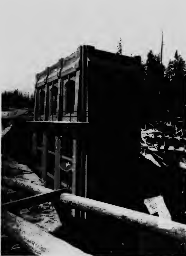
Coquitlam-Bunizen Development. Intake Valve House, Plant No. 2, Lake Bunizen.
